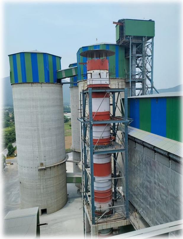
Bag house chimney
