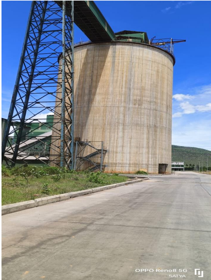
Clinker Storage Silo
