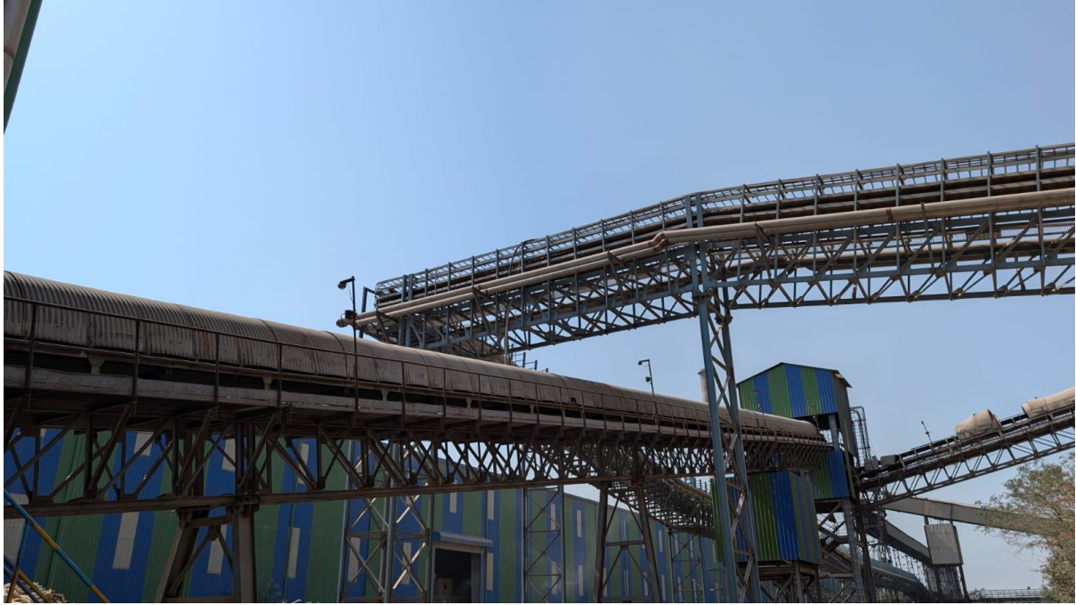
Liquid AFR Feeding System Line-1 & 2
