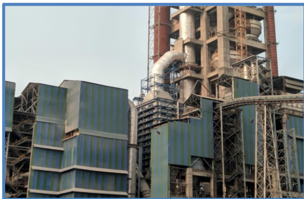
Pre-Heater Boiler (PH Boiler)
