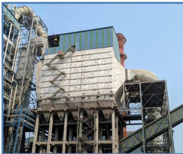
ESP for Clinker Cooler
