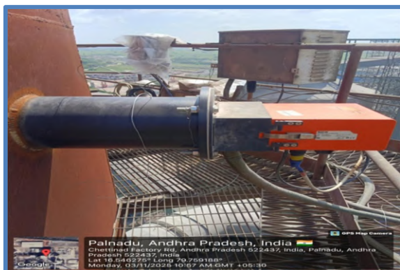
PM CEMS for Clinker Cooler ESP Stack
