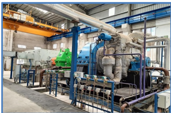
Steam Turbine Generator (STG)
