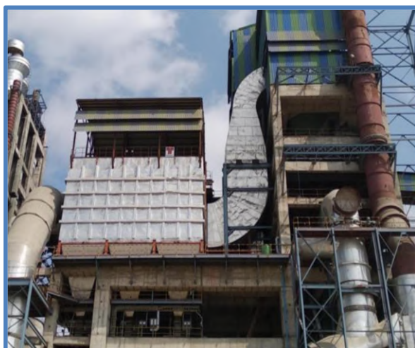
Bag House for Cement Mill
